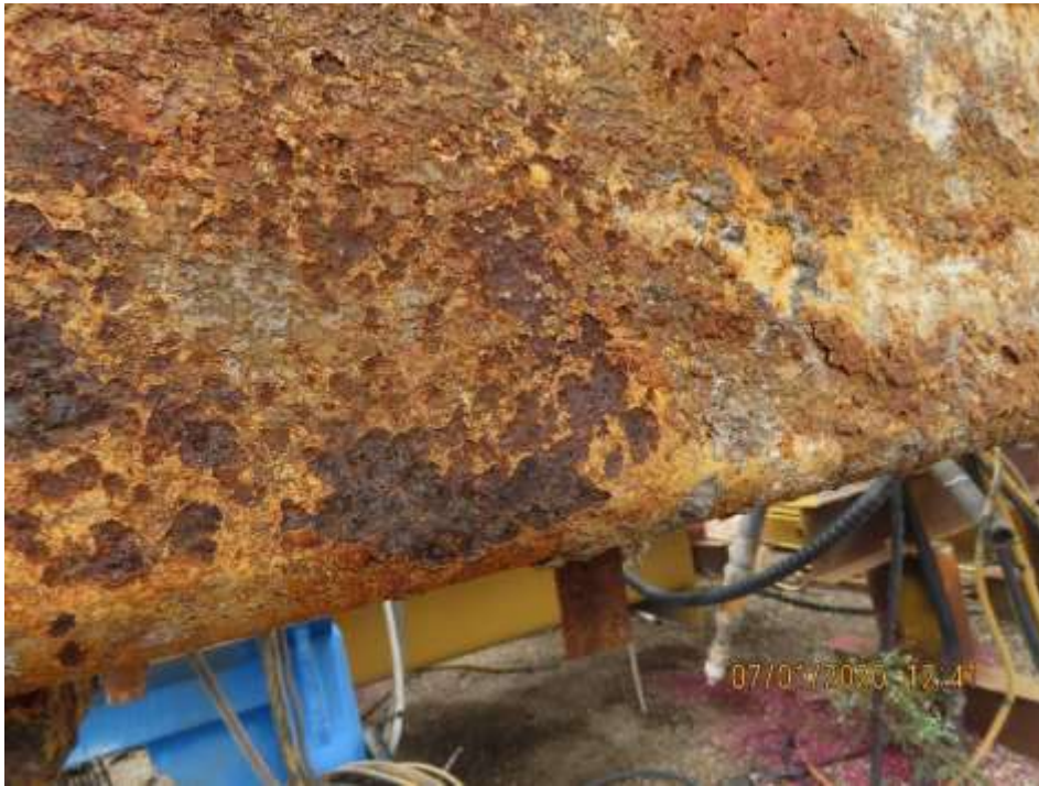
PHOTOGRAPH NO. 9 - Caterpillar 6060 excavator superstructure - corrosion detected on left hand side rail.
